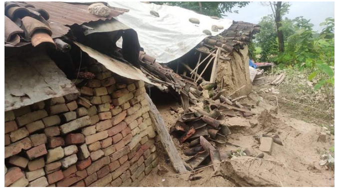
Flood damaged home in Nawalparasi, Lumbini. Source: UNICEF Nepal
